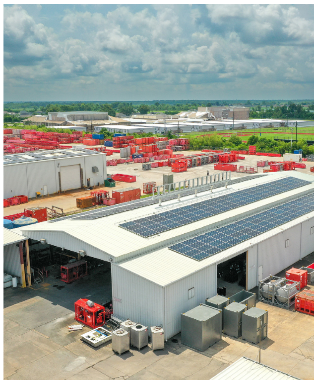
A solar photovoltaic system atop the SES Energy' facility in Houma, Louisiana
